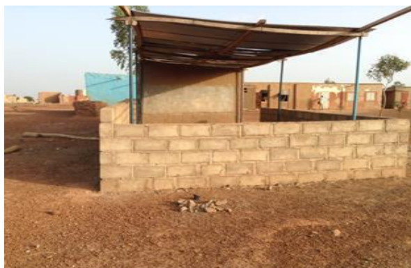
Toilet for students
